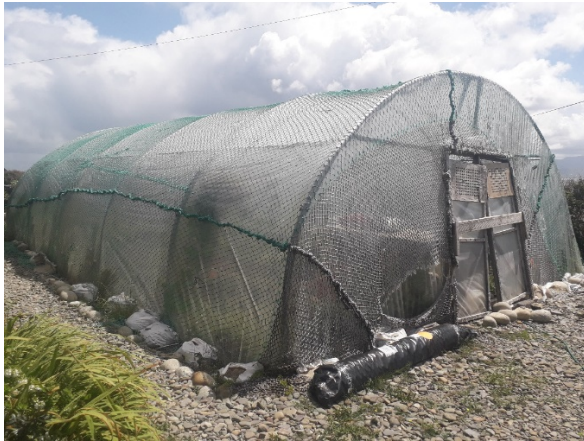
Clare Island Community Polytunnel plastic in need of replacement.
